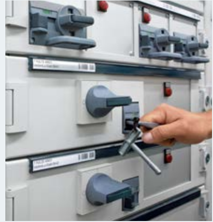
Simple and safe operation of the withdrawable units with the doors closed
