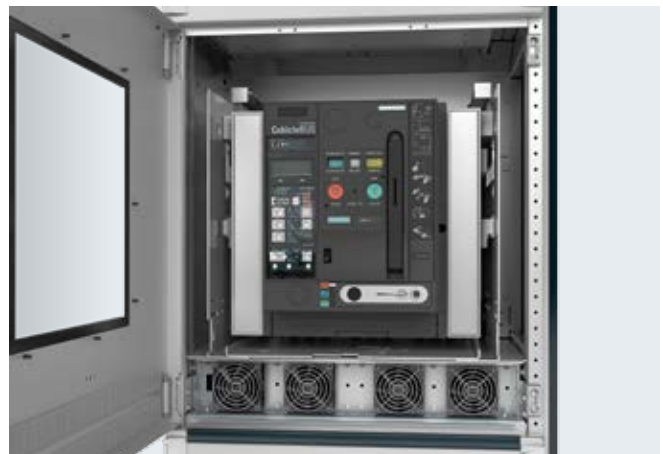
Cooling system with fans underneath the 3WL circuit breaker
